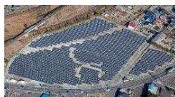
Solar power plants
